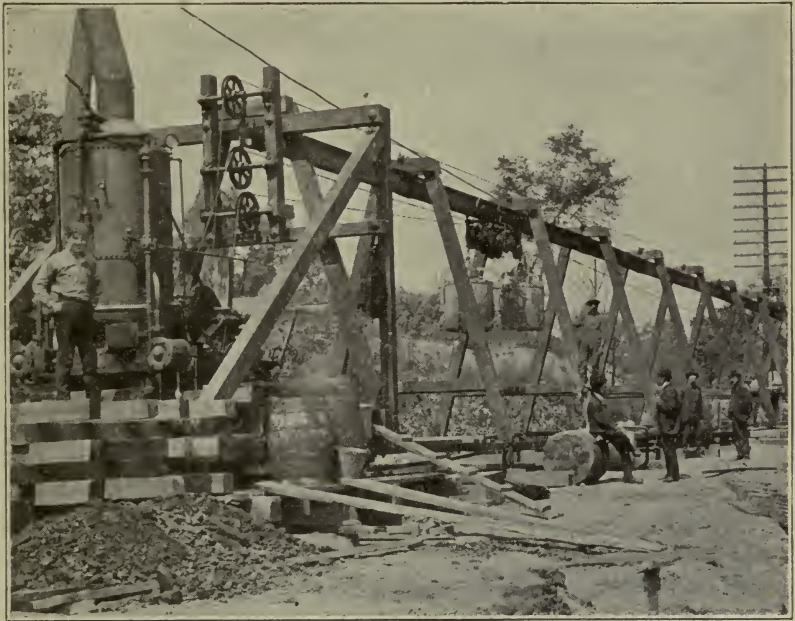
Fig. 70. Trestle Cable Excavator on Sewer Trench Construction Courtesy of Carson Trench Machine Company, Boston, Massachusetts
